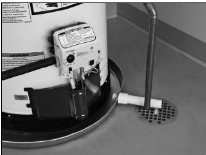
Figure 23 - Metal drain pan piped to drain.
