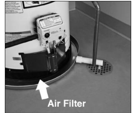
Figure 24 - Filter attached to water heater.
