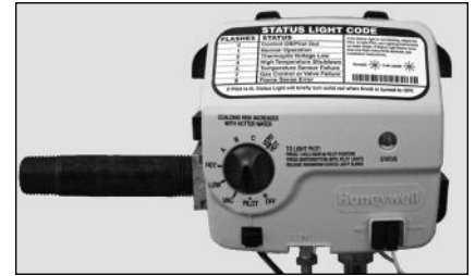
Figure 56 - Gas control/valve with threaded pipe.
