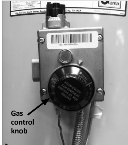
Figure 17 - Turn gas control/temperature knob OFF.
